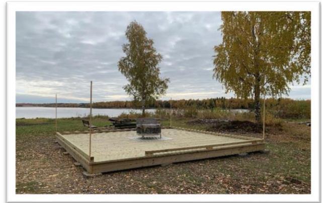
At Vassholmen in Kalix the foundation has been laid for an accessible barbecue area within the LONA project.
